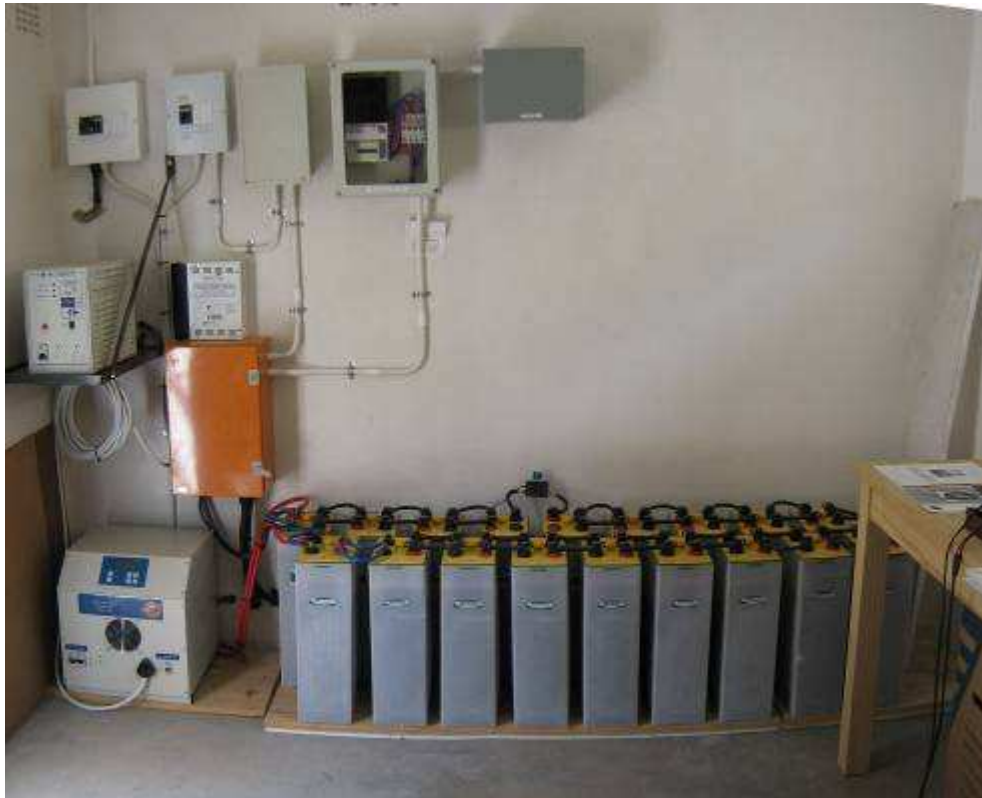
Figure A.5: The control room consisting of the battery bank (18 x 2V, bottom right), inverter (6 kW, bottom left hand corner) and other electrical equipment
